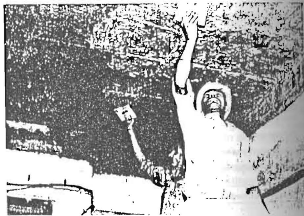
Fig 3 IPN coating application on a badly damaged ceiling in a urea plant
