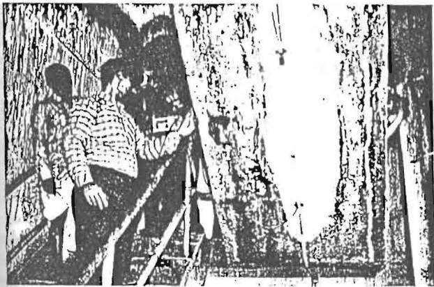
Fig 6 Urea attack on a staircase slab
