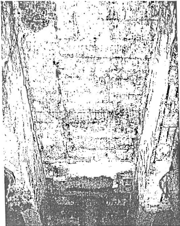
Fig 8 Corrosion distressed slab
