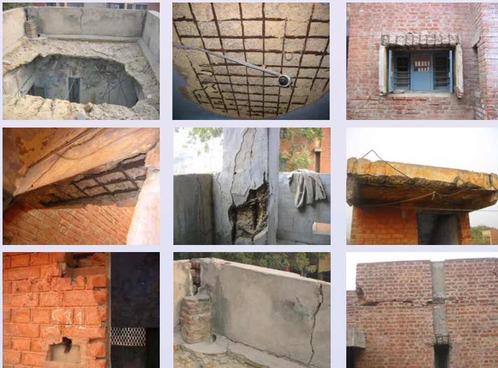
Photos showing damages in slabs, roof slabs, columns, lintels, munties, parapet walls etc.
