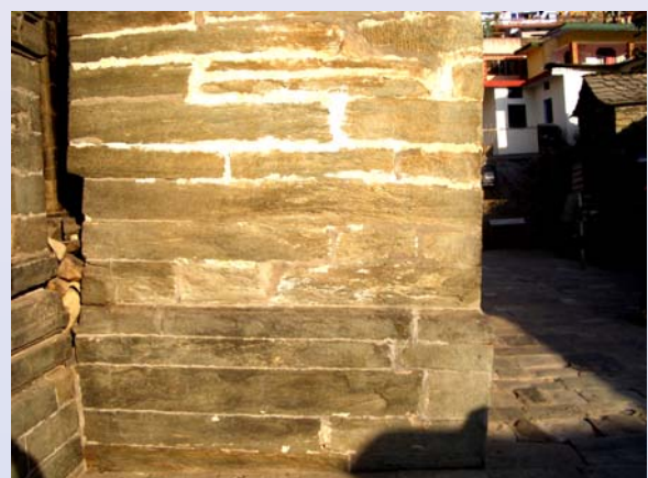
Fig.14-Indication of settlement and Tilting
