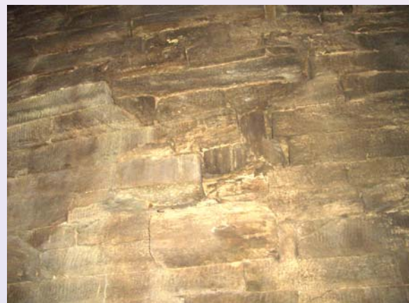
Fig.13-Indication of Water Seepage
