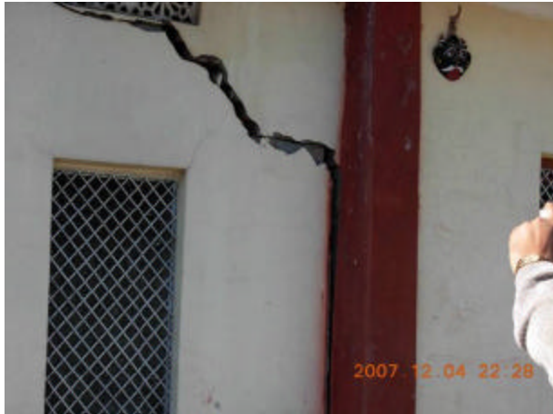
Figure 8. A major crack in one of the houses
