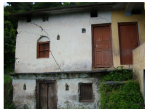
Figure 2 Road subsidence & damaged houses
