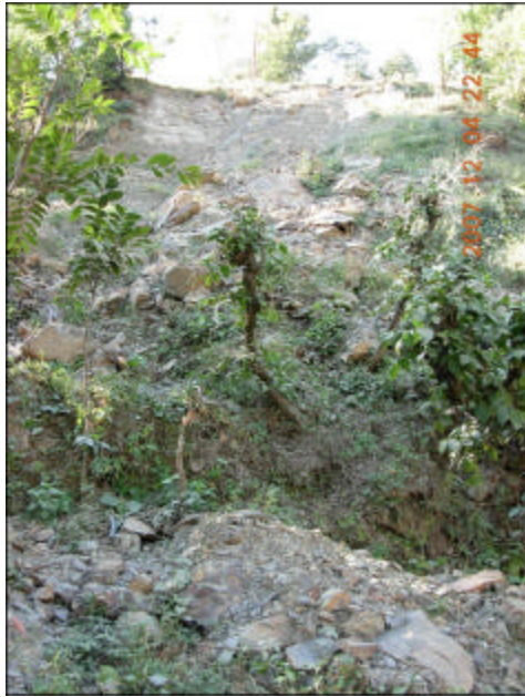
Figure 3. A small landslide on down hill slope
