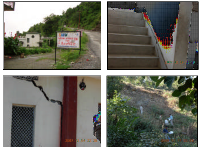
Fig. 3. Damaged houses and local slope failure
