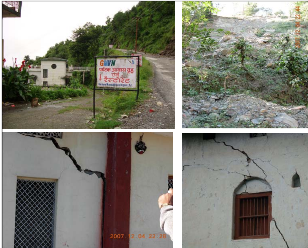
Figure 2 Indications of slope instability manifested by cracks in houses, road subsidence & slope failure
