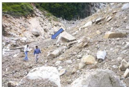
Figure 7. Debris on uphill slope above the road.
