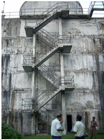
Figure 5 A deteriorated wall of cooling tower.
