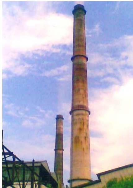
Figure 7 Deterioration of outer surface of concrete chimney
