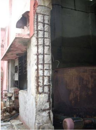
Figure 4 A column showing extreme deterioration due to corrosion in a DM Plant
