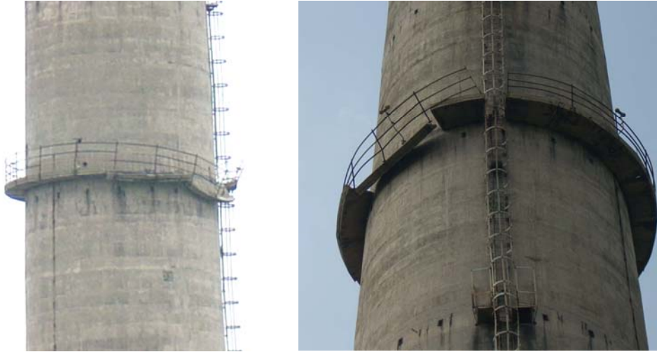
Figure 8 Damaged platforms of the chimney
