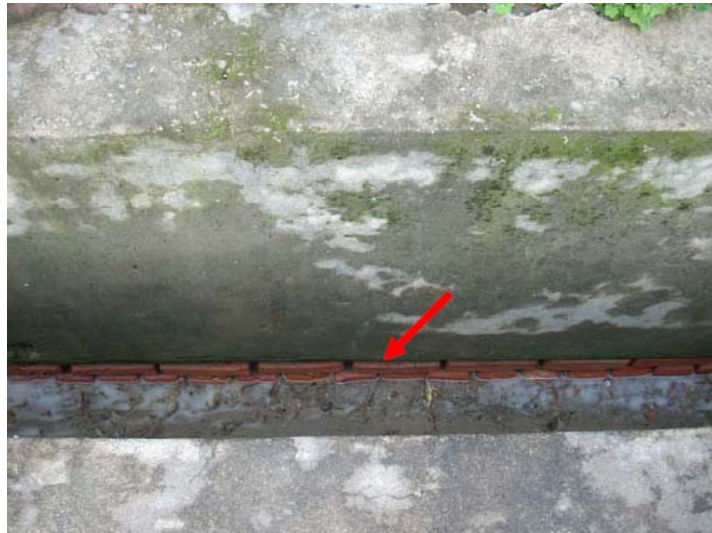
Figure 3 Erosion of plaster in effluent drains
