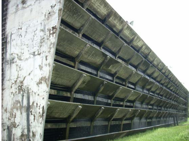
Figure 6 Another view of the cooling tower.
