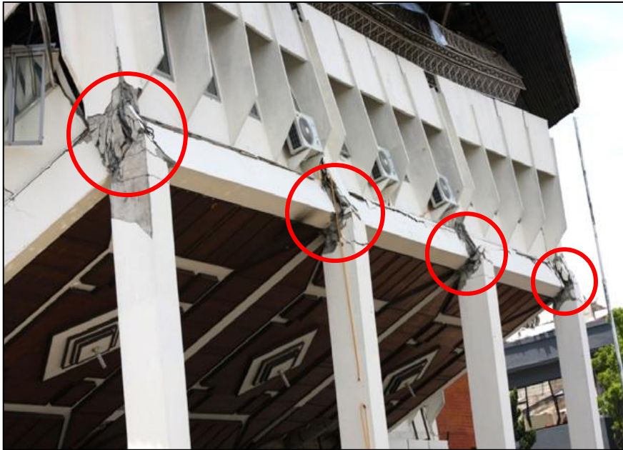
Figure 2.6: Failure of beam-column joint (Sengupta et al., 2013)
