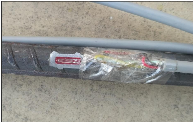
Figure 5.15: Strain gauge at the surface of reinforcement bar near the top concrete surface end (SG1)
