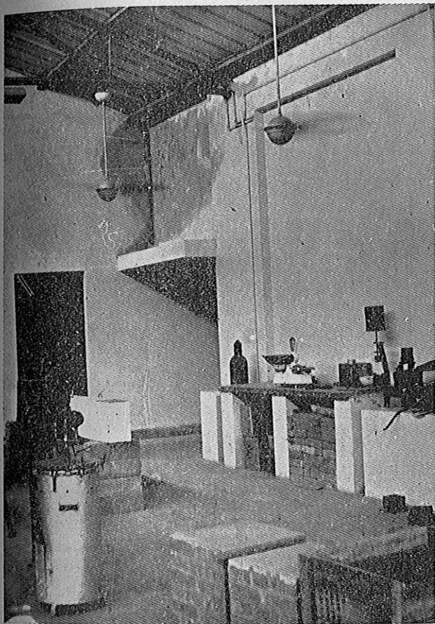
Fig. 2. Dampness at junction of wall with roof
