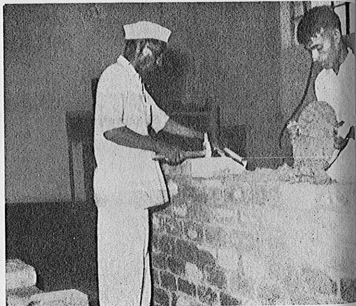
Fig. 2 Wall panel with modular blocks under construction showing supply of mortar directly on the panel.
