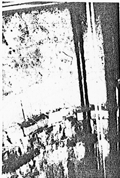
Fig 8 PHOTOGRAPH SHOWING DISLODGING AND DISINTEGRATION OF ACID AND HEAT RESISTING BRICKS ABOVE 70M LEVEL.
