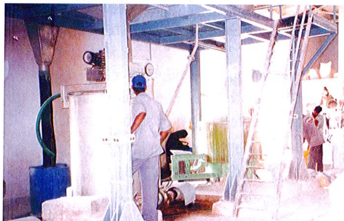
Fig. 2: Phosphogypsum Beneficiation Plant (84 Tpd) Set Up At M/s Orissa Gypsum Ltd., Cuttack, India
